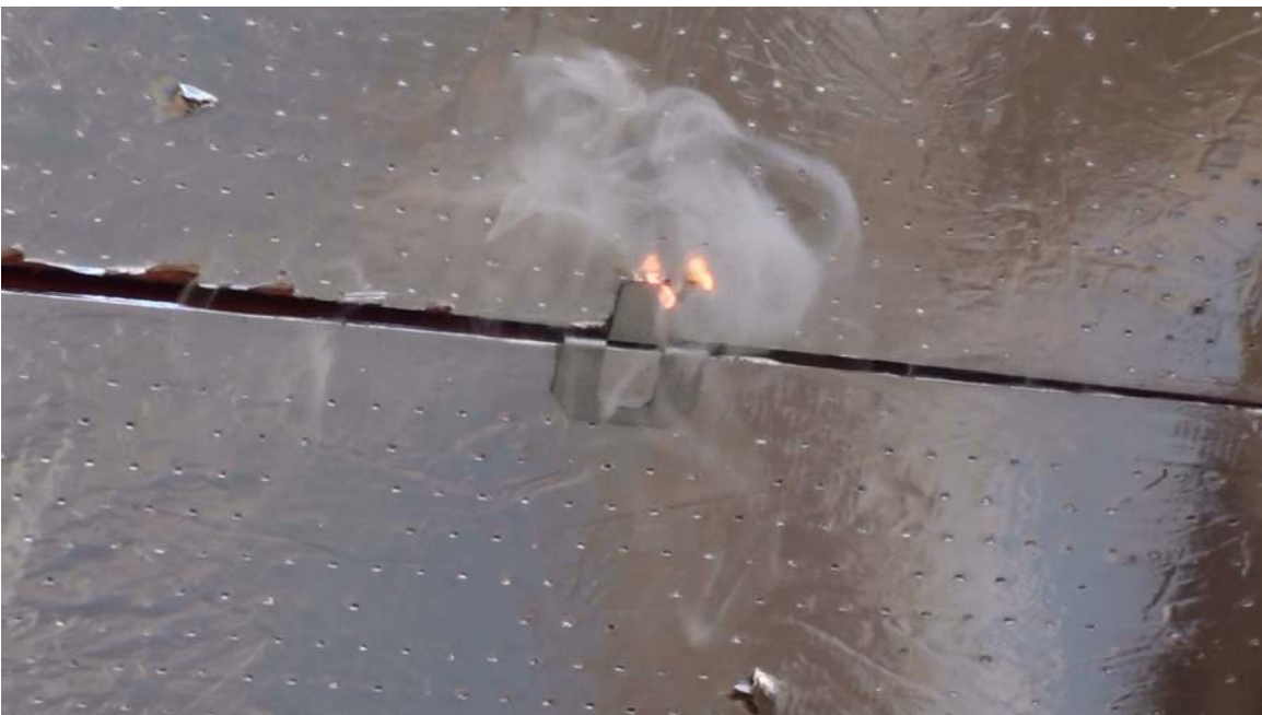
PHOTO #10 Plywood Clip on an Actual Roof Section – Approximately 50 Amps. (Note that it is the barrier material which is igniting. This is because the current in the foil is “funneled” near the clip, thus the current density is highest near the clip)
