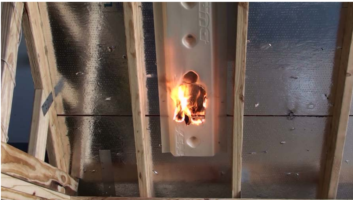
PHOTO #11 Underside of Roof Deck – With Soffit Vent Channels Installed Radiant Barrier was Energized with 12 volts @ 50 Amps
